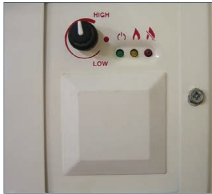
Adjust the temperature of the boiler water by turning the boiler control thermostat.
