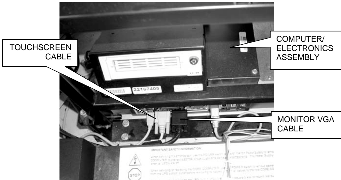
Figure 24 - Touchscreen and VGA Cables
