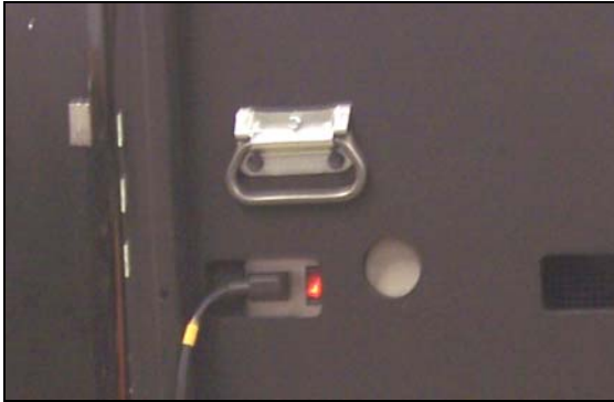
Power Distribution Box - main switch with Circuit breaker
